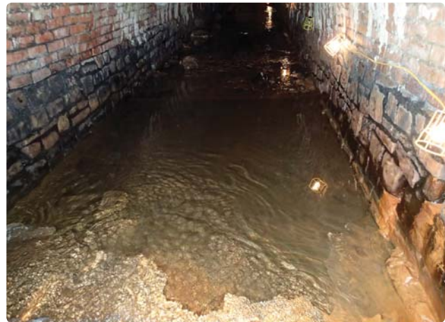
Typical scoured invert area in Nant Tysswg culvert, prior to preparing for repair.
