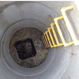
New manhole access constructed to enable concrete pump works at Nant Tysswg culvert.
